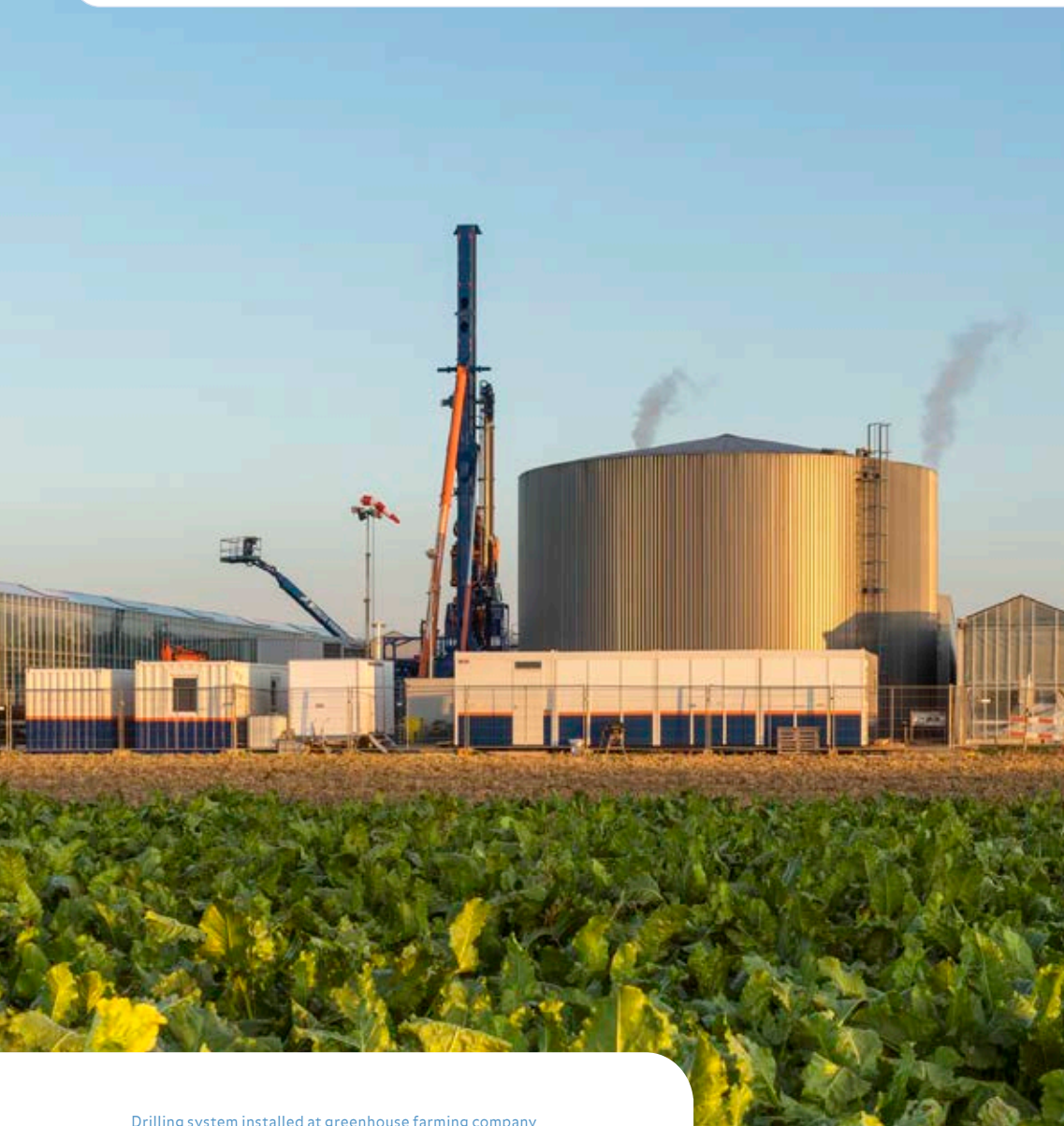
Drilling system installed at greenhouse farming company GreenBrothers in Zevenbergen. The aubergine farm is supplied with sustainable energy in the form of low temperature geothermal heat – a first!
