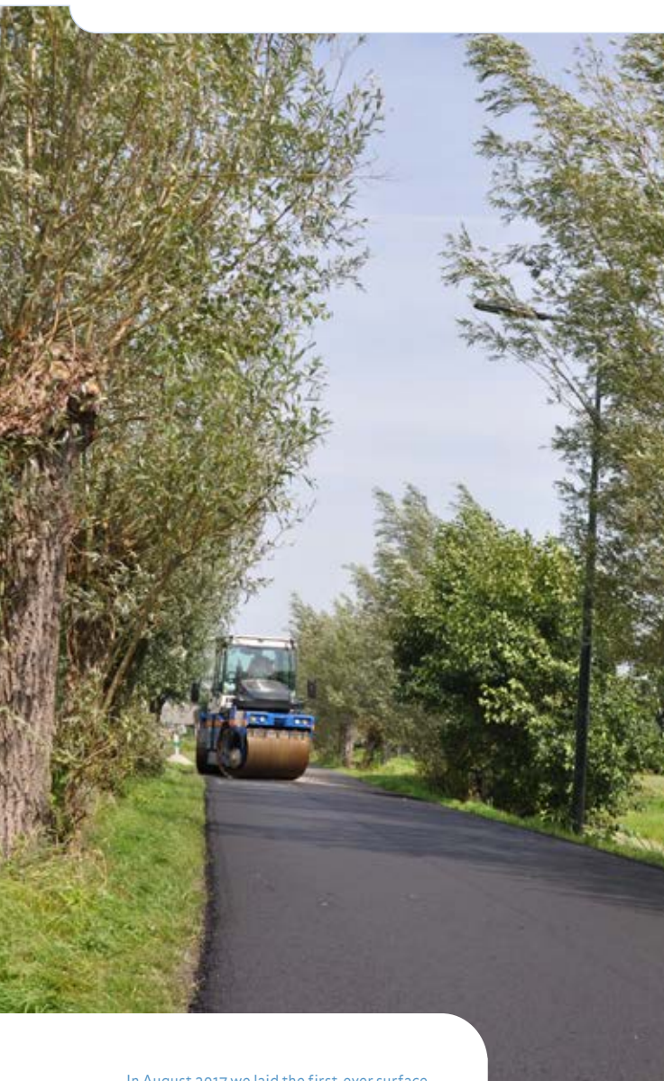
In August 2017 we laid the first-ever surface made from 100% recycled asphalt in a lane for motorised traffic in Ouderkerk aan den IJssel.
