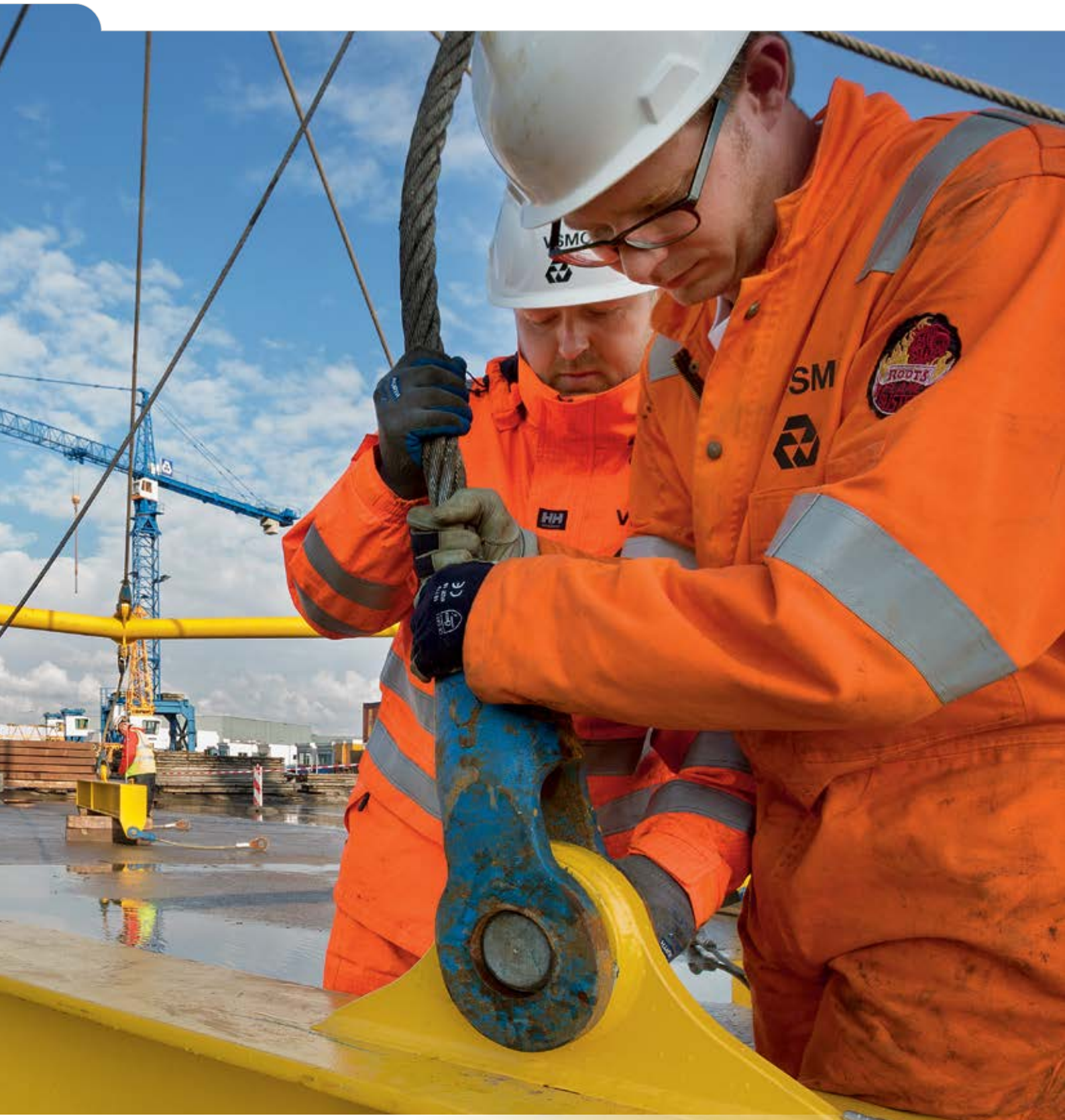
Two vsmc employees are working on a hoisting structure that can be used to place two cable pans aboard a cable-laying ship or barge. vsmc and vsm were responsible for the design and construction of the hoisting structure and the cable pans.
